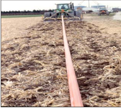
Figure 7. Till the soil 3 to 5 inches deep or 3 inches below the depth of injection to disrupt macropores. (Photo courtesy of Jon Rausch, The Ohio State University)
